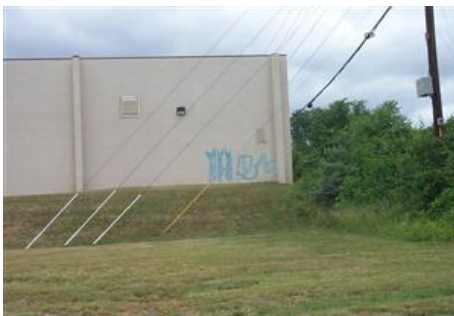
This graffiti was not removed as soon as it was discovered.
